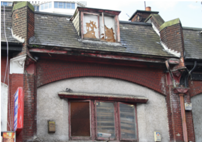
This building is in an extremely dilapidated condition due to lack of maintenance.
