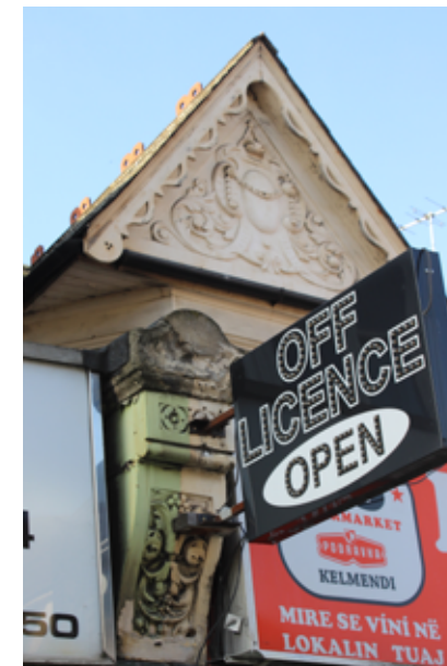
Surviving but damaged historic shopfront corbels often with inappropriately attached projecting signs and pigeon spikes.
